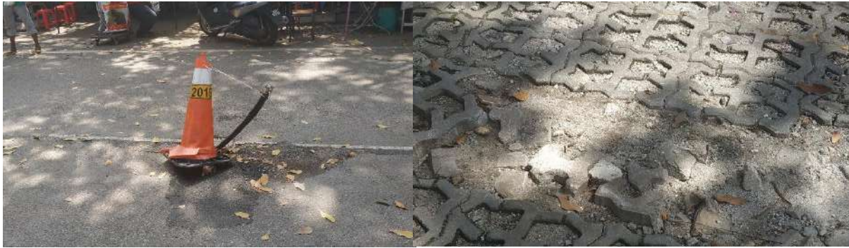
Figure 11: The traffic was caused by bazaar activities which narrow the roadway which also have uneven surfaces.
