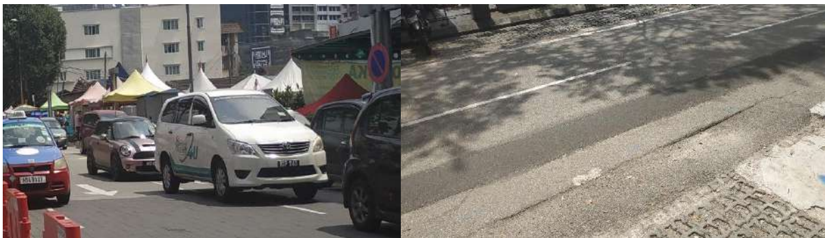
Figure 10: There are defects in the middle of the roadways and defects in tiling on the parking lots.
