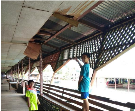
Ceiling destroyed due to act of vandalism. (picture taken during site visit in Kampung Kaban, 6th November 2018)
