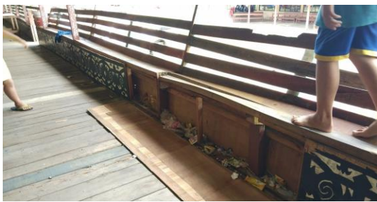
Removed ornament panel and cavity filled with trash. (picture taken during site visit in Kampung Kaban, 6th November 2018)
